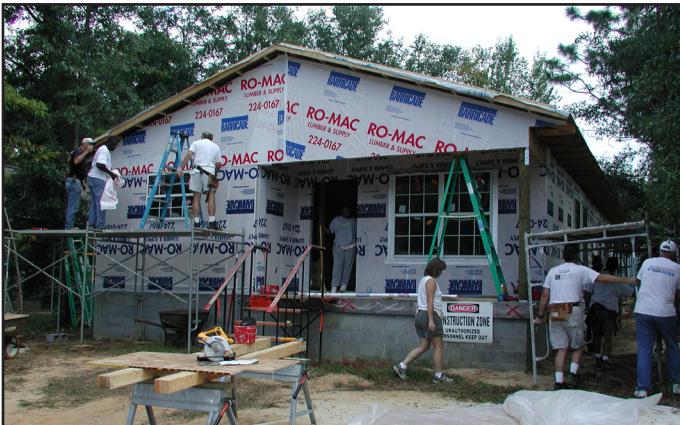
This photo, taken from a previous build, shows how a few determined volunteers paired with the necessary supplies, really can build a beautiful home. If you have the time, Habitat will provide the place to volunteer! (photo by Marti Chumbler)
