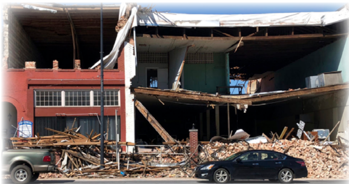
Brick facades were blown from building fronts in downtown Marianna.
